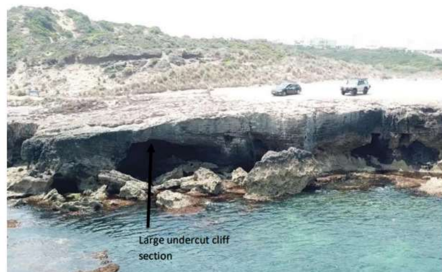
Figure 12: Carpark at the end of Joy Terrace with cliff undercut sections visible
