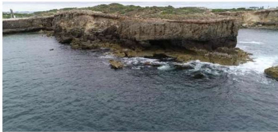
Risk Zone 5 - Cliff Undercutting
