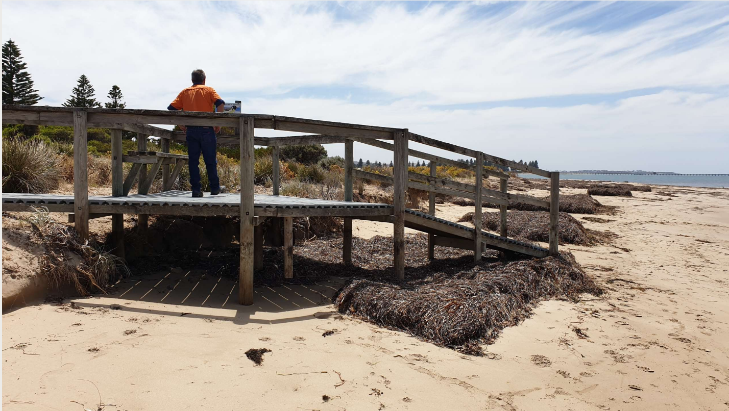
Recent erosion left the beach access way stranded on the beach, Kent Reserve, Victor Harbor, 2021.
